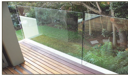
Figure 5 - Structural Balustrade A: Non-compliant above 1 metre fall height. (Source: www.elitebalustrades.com.au )
