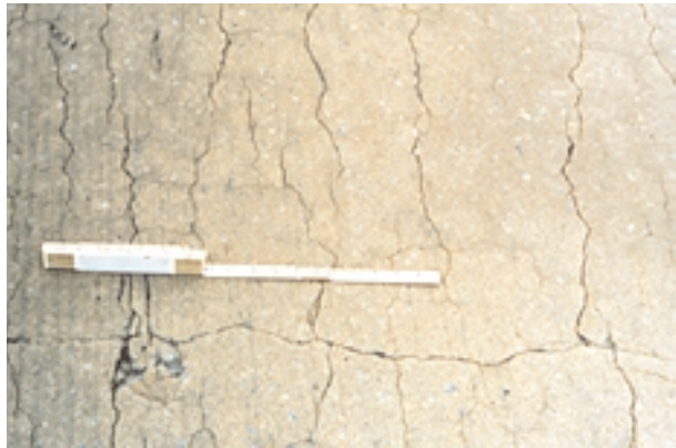
Fig. 5-20 (top and bottom). Cracking of concrete from alkali-silica reactivity. (69549, 58352)
