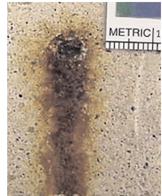
Fig. 5-19. Iron oxide stain caused by impurities in the coarse aggregate. (70024)
