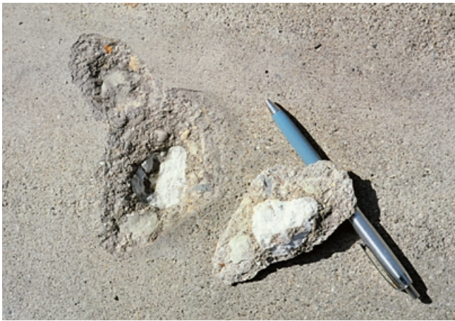
Fig. 5-18. A popout is the breaking away of a small fragment of concrete surface due to internal pressure that leaves a shallow, typically conical depression. (113)
