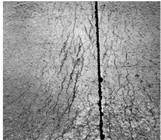
Fig. 5-15. D-cracking along a transverse joint caused by failure of carbonate coarse aggregate (Stark 1976). (30639)
