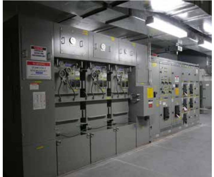
Figure 14. Triplex Indoor Power Center comprised of energy efficient and low noise single-phase substation transformers in a ganged setup.
