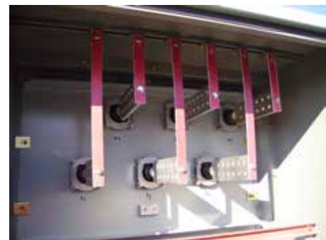
Figure 11. 12-pulse application with bushing supports.
