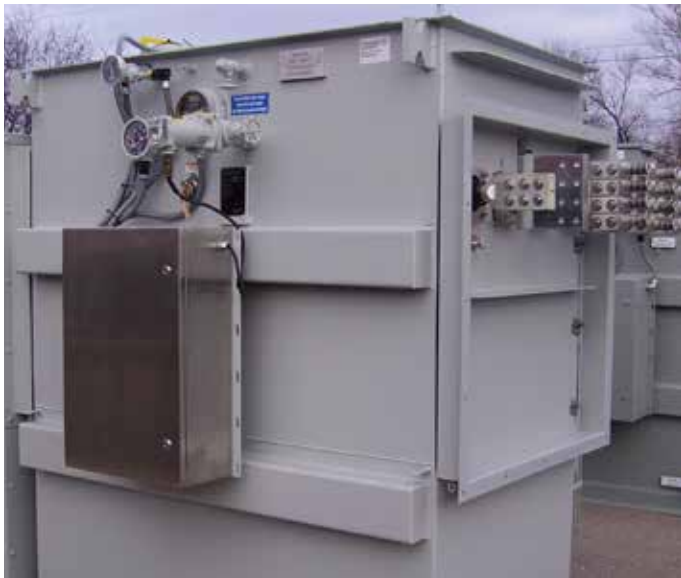
Figure 13. Substation transformer with customer-specific coordination and accessories.
