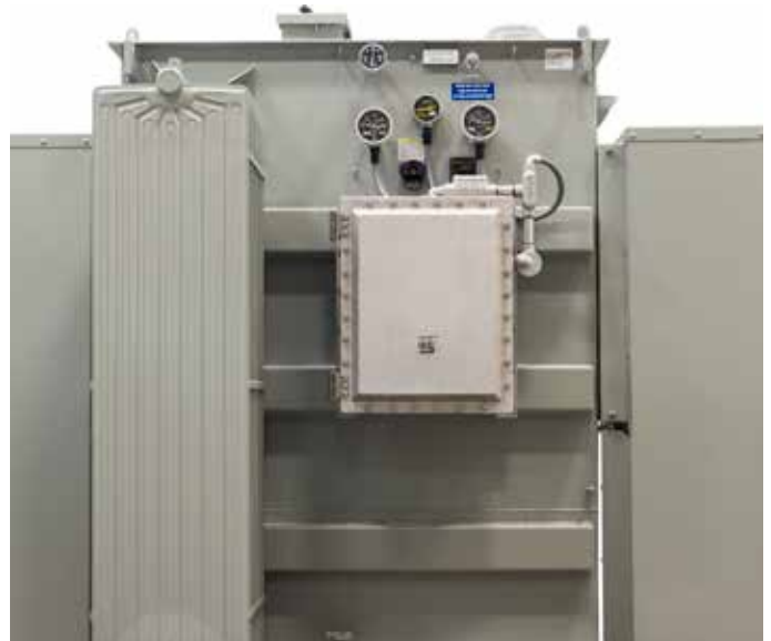
Figure 15. Class 1 Div 2 hazardous duty substation transformer.
