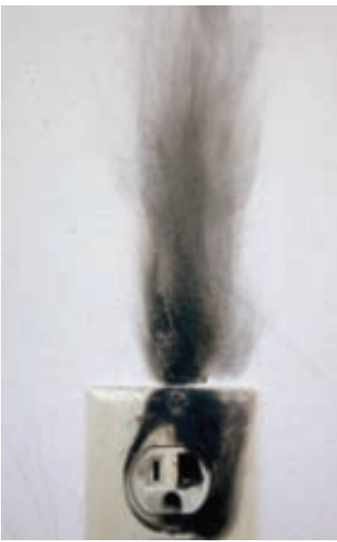
Figure 4-15. The charred electrical outlet and the surrounding burn pattern indicate an electrical fire.
