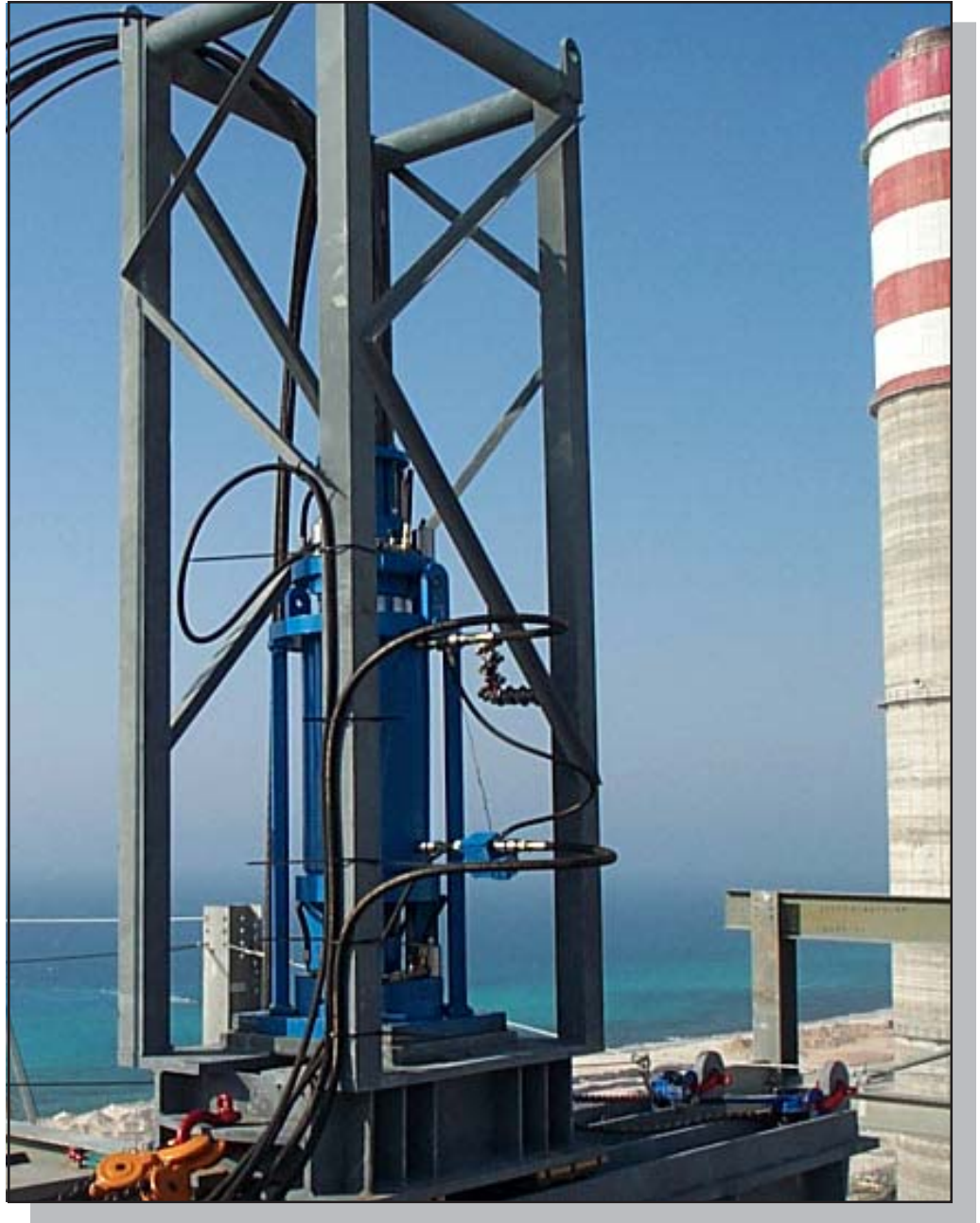
Figure 5.8-1 Strand Jack System
