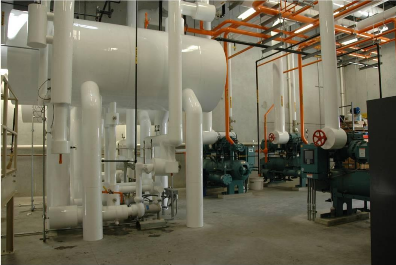
Ammonia Recirculator Package
