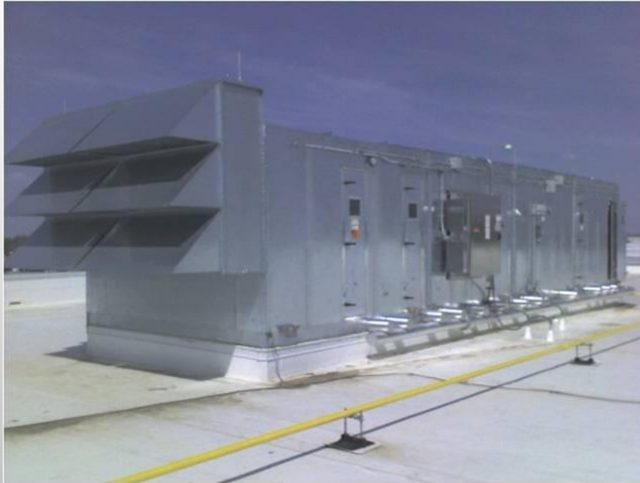
Rooftop Air Unit for Cooling and Make-up Air
