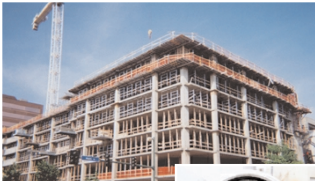
Fig. 9-1. Trial batching (inset) verifies that a concrete mixture meets design requirements prior to use in construction. (69899, 70008).
