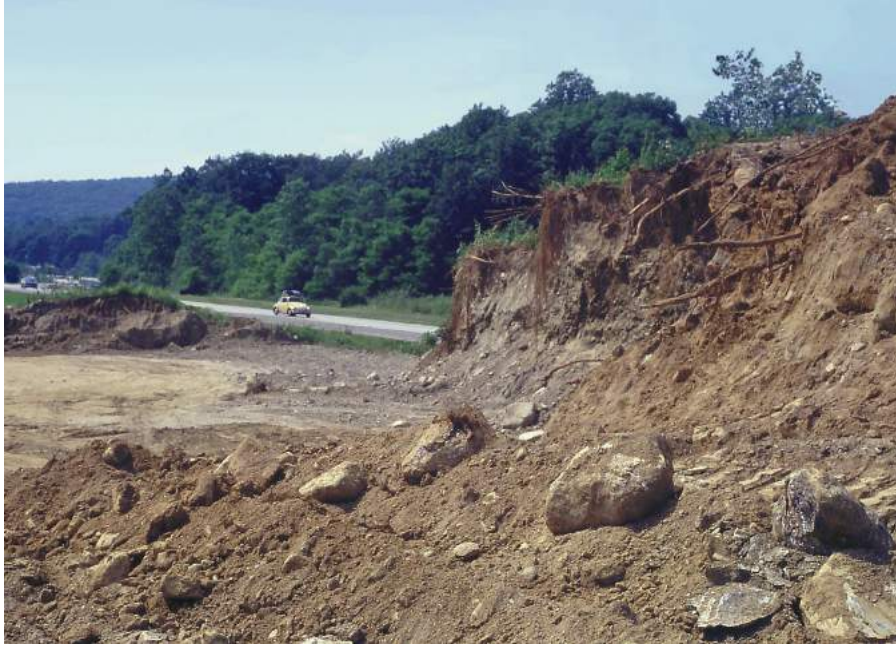
FIGURE 8-13. This construction site in Westchester County, New York, contains unsorted sediments deposited by glacial ice.
