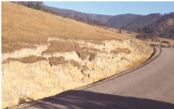
FIGURE 8-4. Mass movement occurred along a slope that was made steeper by road construction and lubricated by water in the soil.
