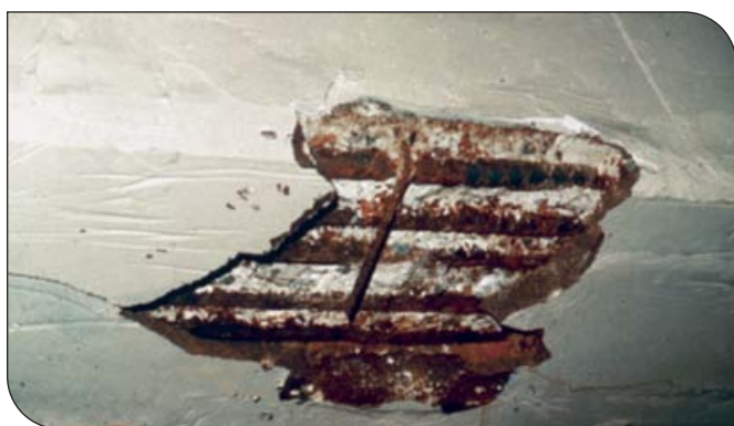
Fig. 6. The damage to this concrete beam, located in a parking structure, resulted from chloride-induced corrosion of steel reinforcement. (IMG25527)
