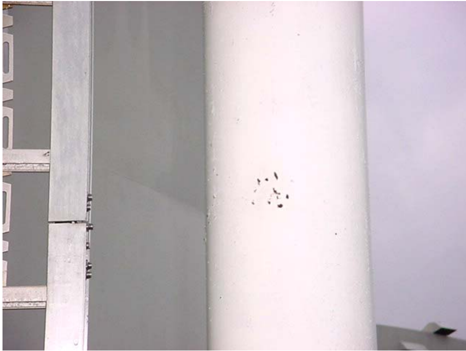
Figure 1. Photograph of peeling paint from pipeline.
