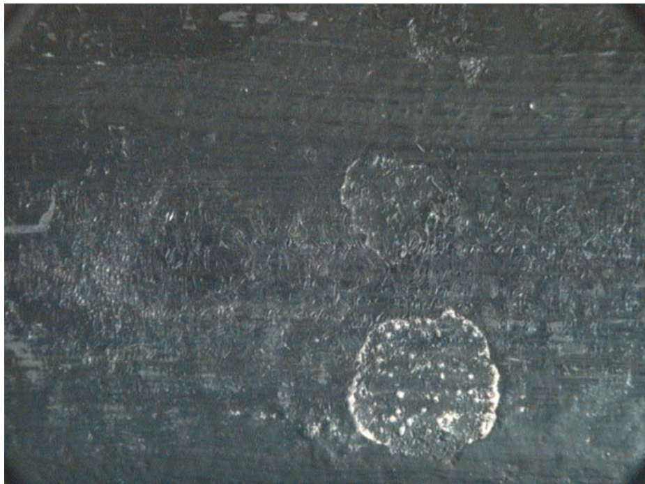
Figure 26. Photograph showing a repaired blister area.
