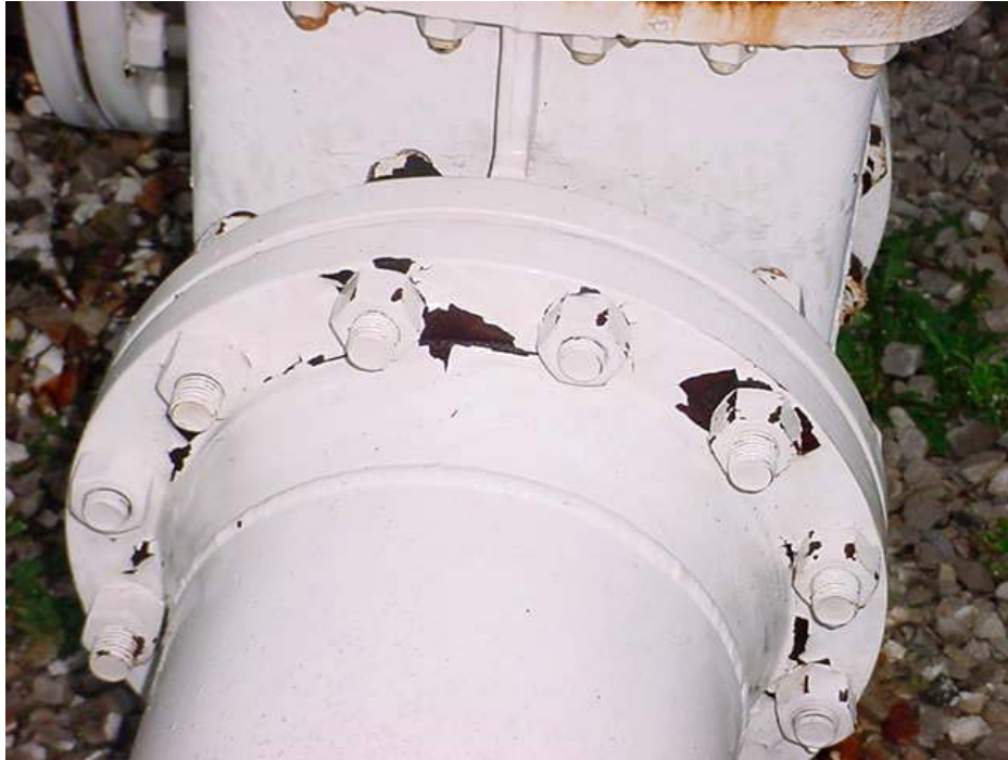
Figure 3. Photograph of peeling paint from flange on pipeline.
