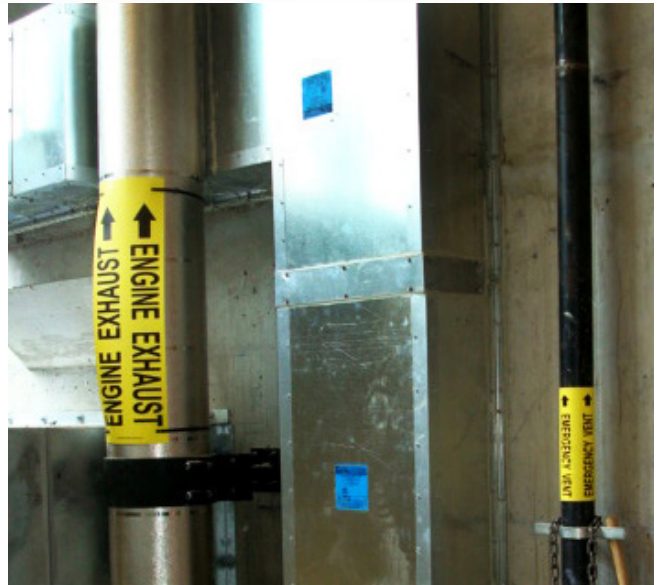
A fire-rated pipe enclosure.
