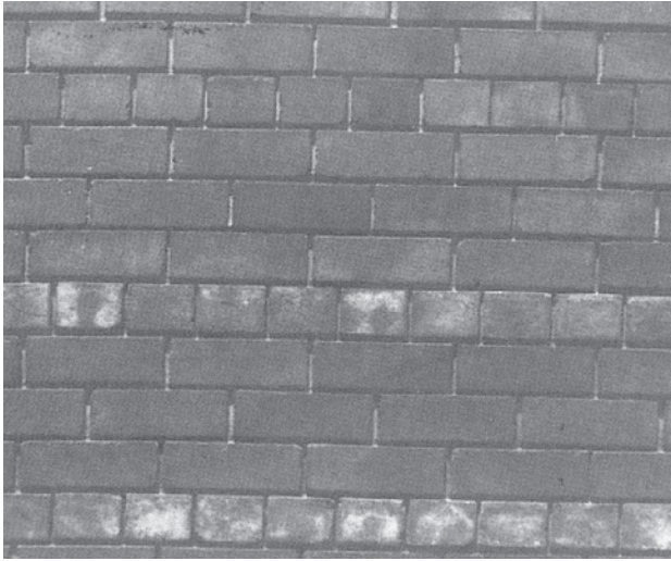
Efflorescence in header courses of a brick retaining wall due to salts conveyed from soil by water.
