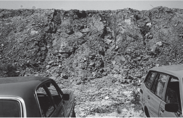
Unretained filling shows effects of water erosion and loose boulders, Excavation is unpredictable.
