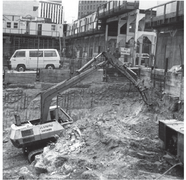
Heavy machinery excavating solid sandstone to a vertical face for a building basement.
