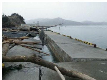
Fishing port pier destroyed by the earthquake and tsunami (Ishinomaki City, Miyagi Prefecture)
