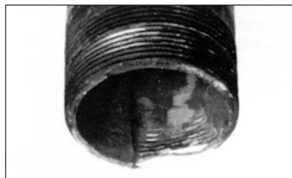
Figure 9-9. CO 2 gas combines with condensate allowed to cool below steam temperature to form carbonic acid, which corrodes pipes and heat transfer units. Note groove eaten away in the pipe illustrated.
