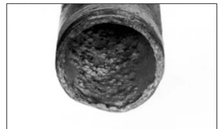
Figure 9-10. Oxygen in the system speeds corrosion (oxidation) of pipes, causing pitting such as shown here.
