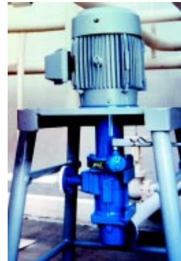
Vertical, Magnetic Drive 3D-250 pump in chemical service - Freeport, Texas, USA
