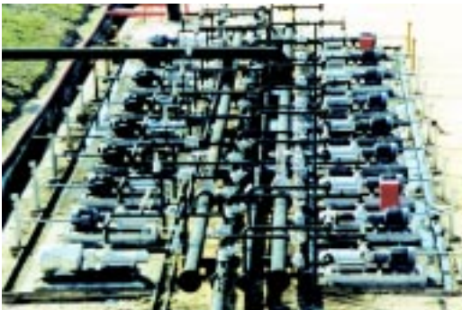
6D series pumps in crude oil service - Pacific Rim
