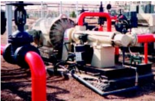
8L and 12D series pumps in crude oil service - Alberta, Canada
