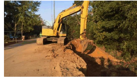
Cleanup activity at the Kerr-McGee Chemical Corp. Superfund site in Columbus, Mississippi. (EPA photo)
