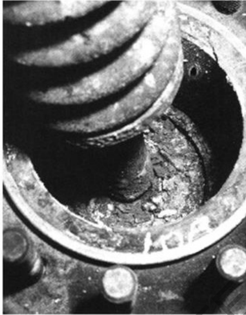
Figure 34 - Moving Parts of Valve Fouled with Iron Sulfide (FeS 2 )
