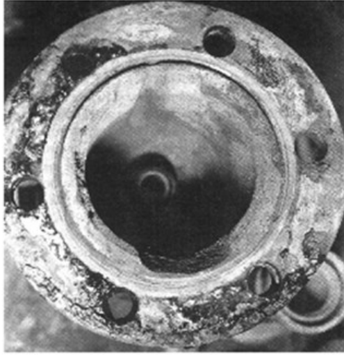
Figure 21 - Acid Corrosion in Carbon Steel Bonnet Caused by Leaking Seating Surfaces
