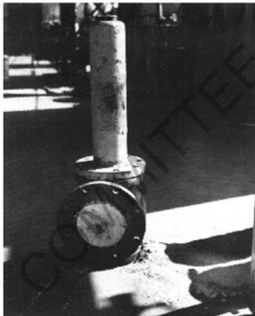
Figure 33 - Outlet Valve Plugged with Deposits from Other Valves in Common Discharge Header
