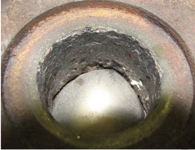
Figure 48 - Rupture Disk Holder Subjected to Excessive Corrosion
