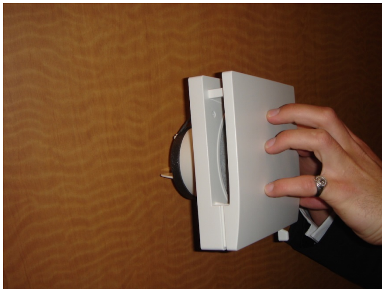
Figure 6. Passive air inlet—Ventilation air can only be introduced into multifamily units by infiltration through exterior walls or directly into the units by ducted supply or passive air inlets (holes in the exterior walls)
