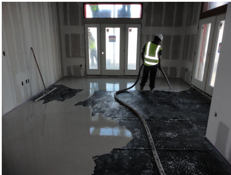
Figure 4. Floor assembly air sealing—Floor assemblies that are soundproofed and fireproofed with liquid gypsum subflooring result in airtight wall assemblies at floor to wall connections
