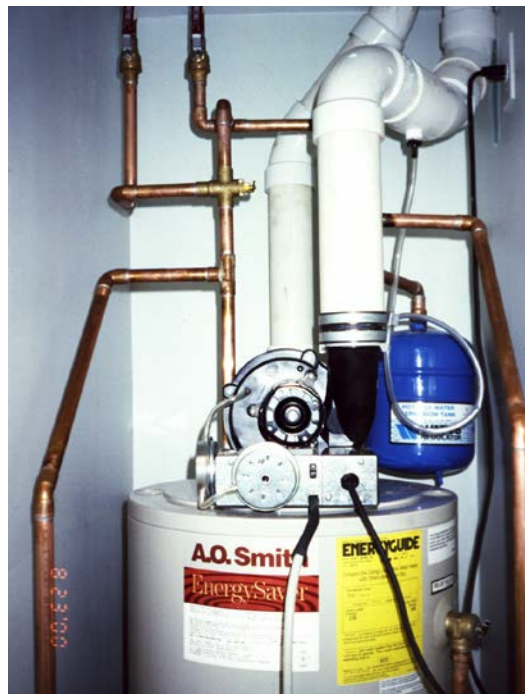
Figure 15. Gas water heater—Gas water heaters should be sealed combustion two-pipe systems vented directly to the exterior with combustion air ducted directly to the water heater
