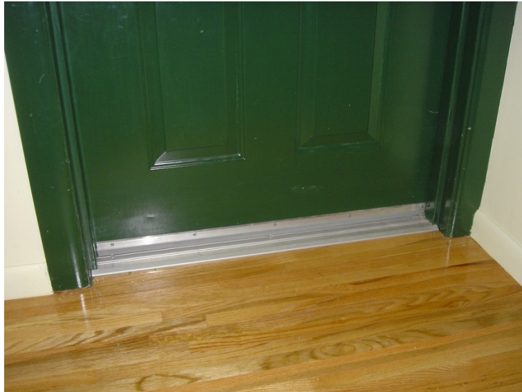
Figure 5. Weatherstripped corridor doors—Ventilation air is prohibited from being introduced into multifamily units from corridors; doors from multifamily units to corridors are typically weatherstripped
