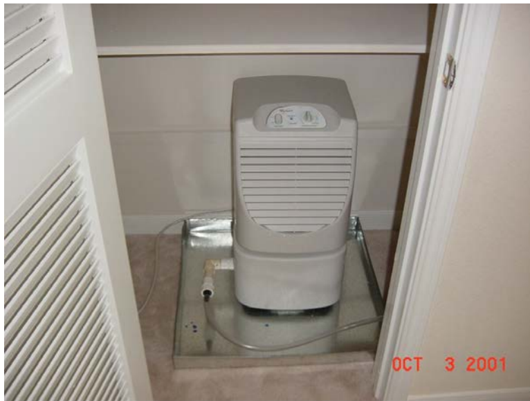
Figure 21. Dehumidifier—Located in closet with louvered door
