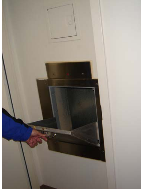
Figure 27. Trash chute—Should be maintained at a negative pressure
