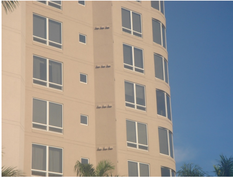
Figure 12. Individual supply and exhaust openings—Multiple exhaust grilles and supply grilles are required
