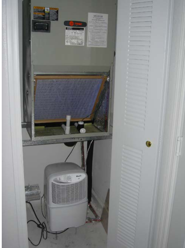
Figure 20. Dehumidifier—Located in return closet
