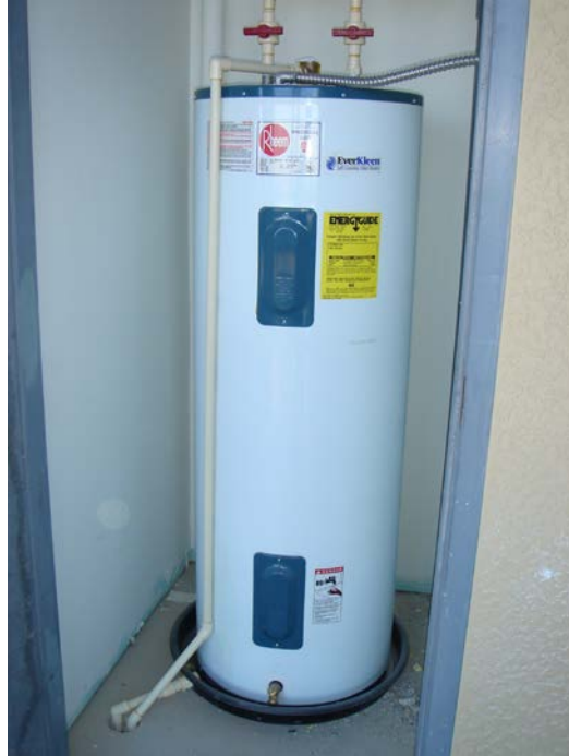
Figure 14. Electric water heater—Electric water heaters do not need to be vented to the exterior, whereas gas water heaters do
