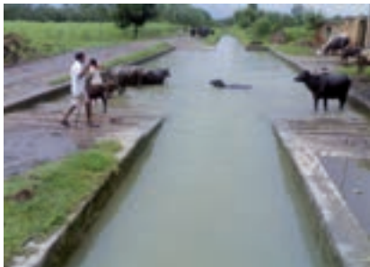
PHOTO 4.1 Cattle ramps on a distribution canal (Main Ganga canal – Uttar Pradesh)
