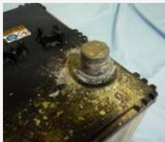
Battery terminal condition Check Looseness, Corrosion
