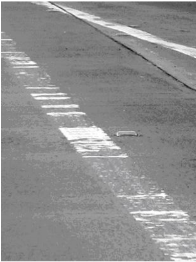
Figure 2-11. Major thermoplastic failure on concrete.
