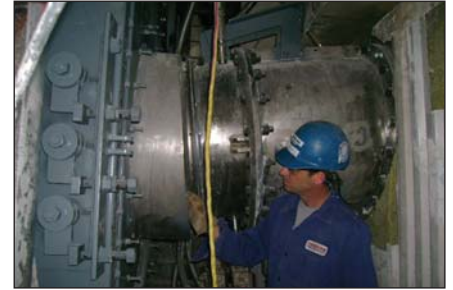
Refractory Lined Bed Transfer Expansion Joints
