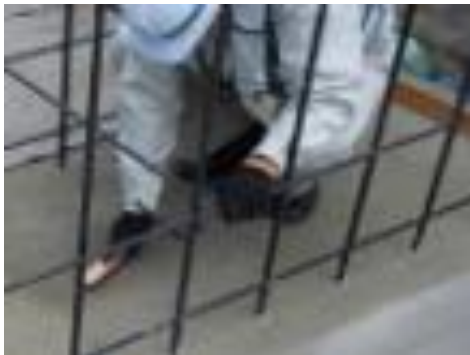
Figure 11.2-2 Treatment of C.J by Wire Brush (Treating after passing a relatively long time)
