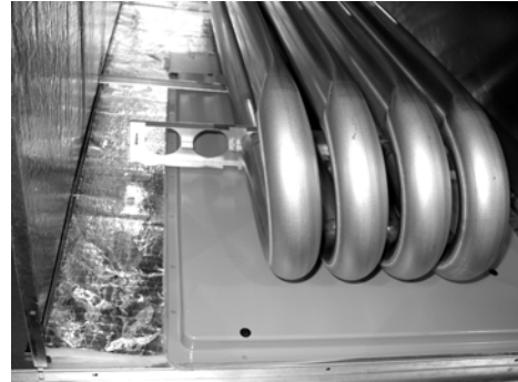
Figure 19: Discharge Panel In Place
