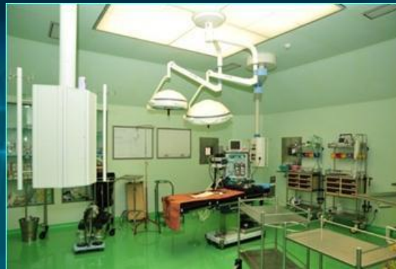
MODULAR OPERATION THEATRE
