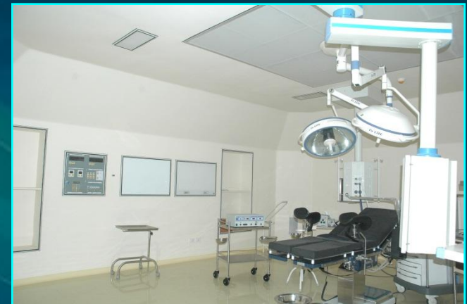
Modular Operation Theatre in JIPMER, Puducherry
