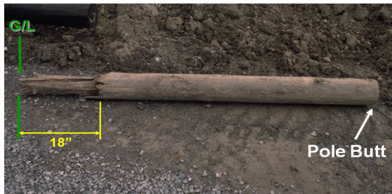
Figure 15 Pole Failure due to Decay in 18 inch decay section (Bingel, 2011)
