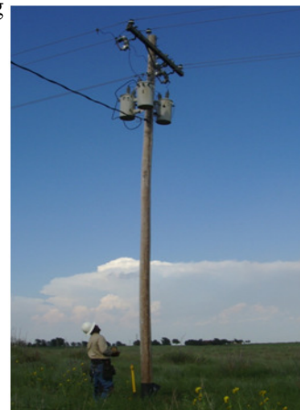
Figure 4 Typical Wood Distribution Pole (Bingel, 2011)
