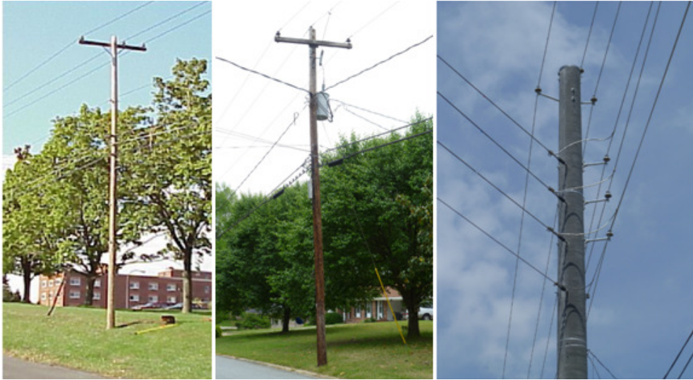
Figure 9: a) Tangent pole (Bingel, 2011), b) Guyed pole (Crosby, 2011), c) Self-supporting concrete distribution pole (Crosby, 2011)
